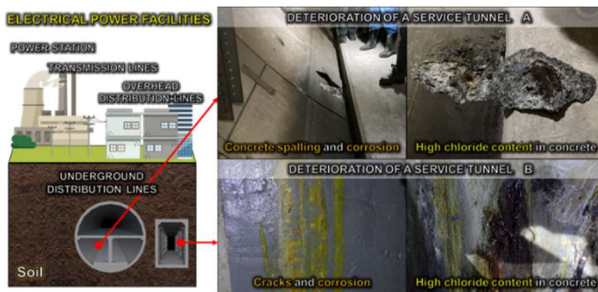
Fig. 1 Deterioration in Reinforced concrete service tunnels
