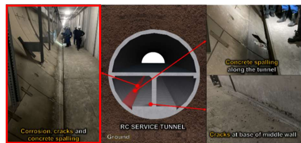
Fig. 3 Deterioration in the left section of the service tunnel
